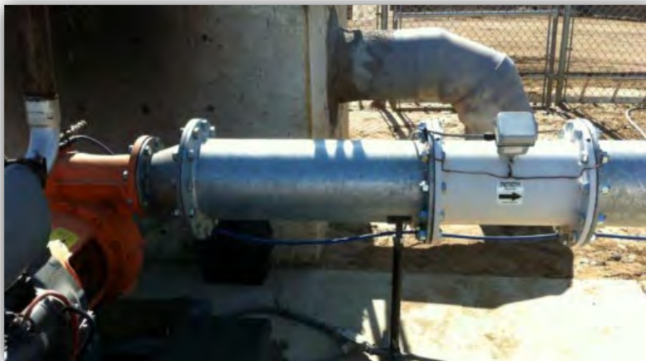
Figure 3: Example of Installed Magmeter in SSJID
