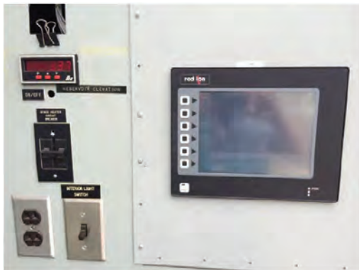
Photo C. Cordell Meter and Data Logger
