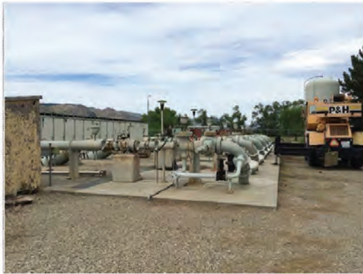
Photo A. Cordell Pump Station
