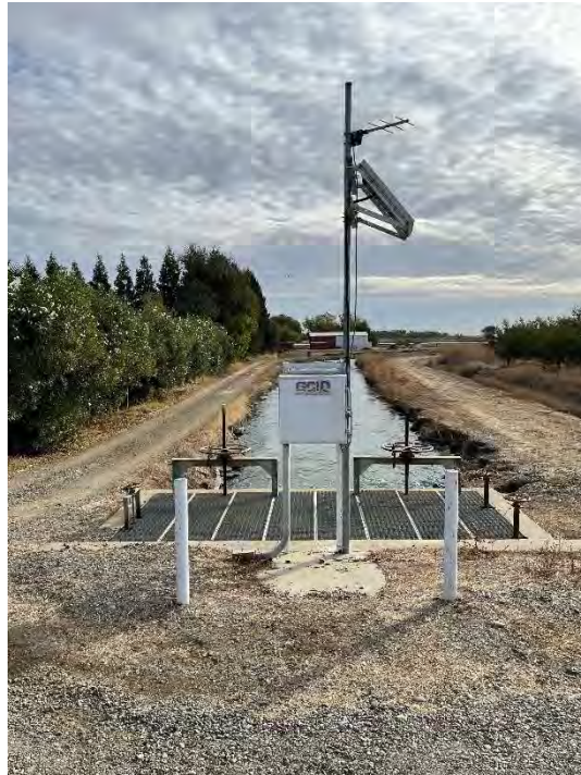
Figure 13. Existing SCADA Integrated Headgate Measurement Site at Lateral 25-1
