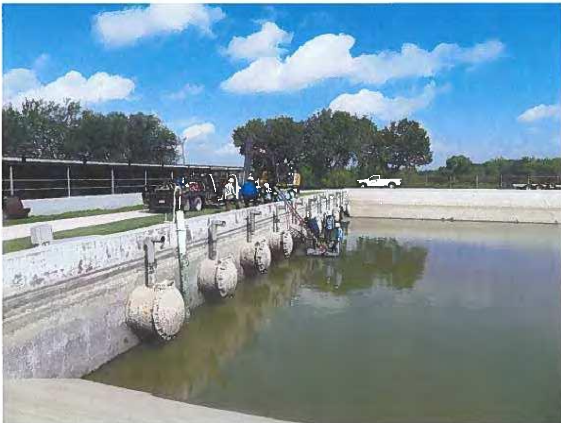
Picture 4. May 27, 2021. The District's crew repairing the hinge of flap valve No.5.
