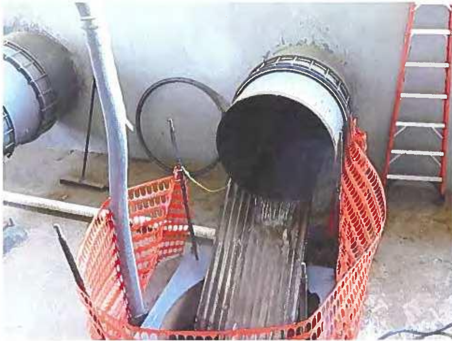
Picture 1. October 18, 2021. Visible backflow from discharge pipe No. 9. The District had remove Pump No. 9 for maintenance. At the time the backflow was directed back to Pump No. 9's base plate opening with the aid of a corrugated metal panel.
