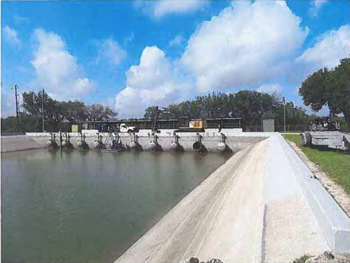
May 27, 2021. HCID 2 River Pumping Plant. In the background visible are the ten 42-inch welded steel discharge pipes and corresponding flap gate. The District's crew was busy repairing flap valve No. 5
