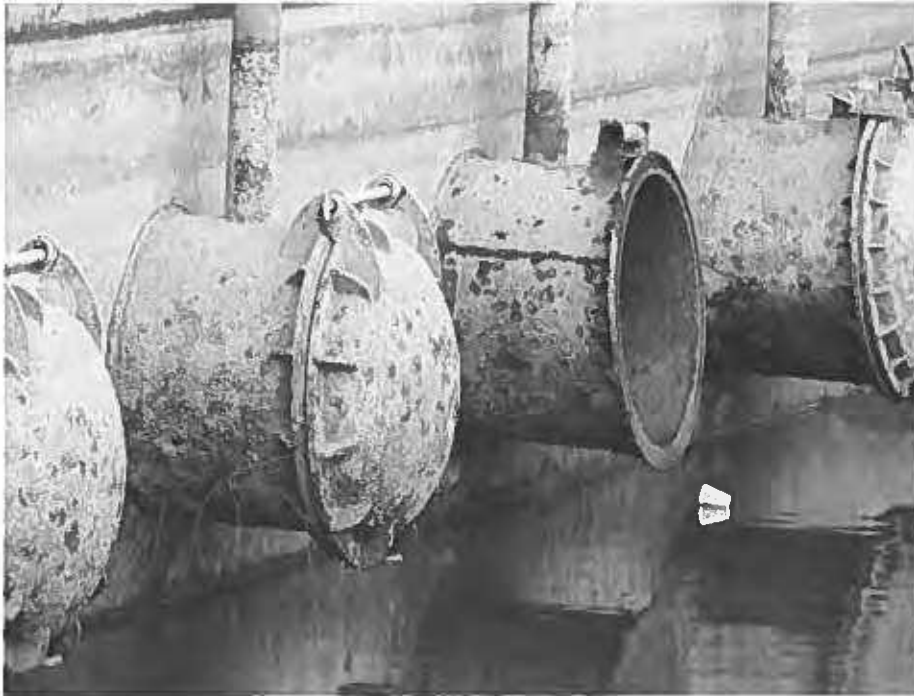
Picture 7. May 27, 2021. Single visible hole in discharge pipe No. 8. The red lead arrow was inserted to point to the hole location. Flap Valve No. 9 was installed the following day. The holes in pipes 9 and 10 are overshadowed and camouflaged.
