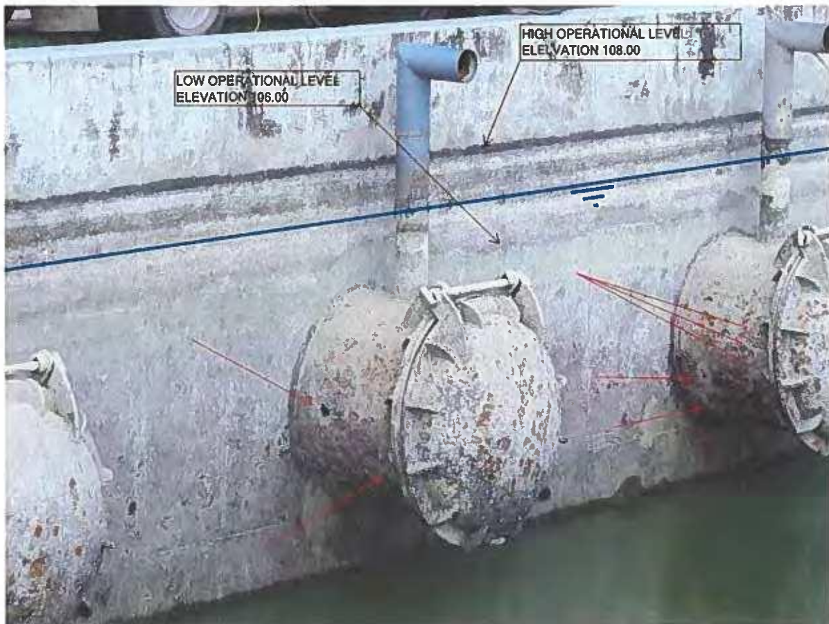
Picture 6. May 27, 2021. Two visible holes in discharge pipe No. 3 and numerous holes in discharge pipe No. 4. The red lead arrows were inserted to point to the hole location. Text boxes were inserted to indicate the Feeder Canal's operational levels. The blue line indicates the mean operational level corresponding to elevation 107.00.
