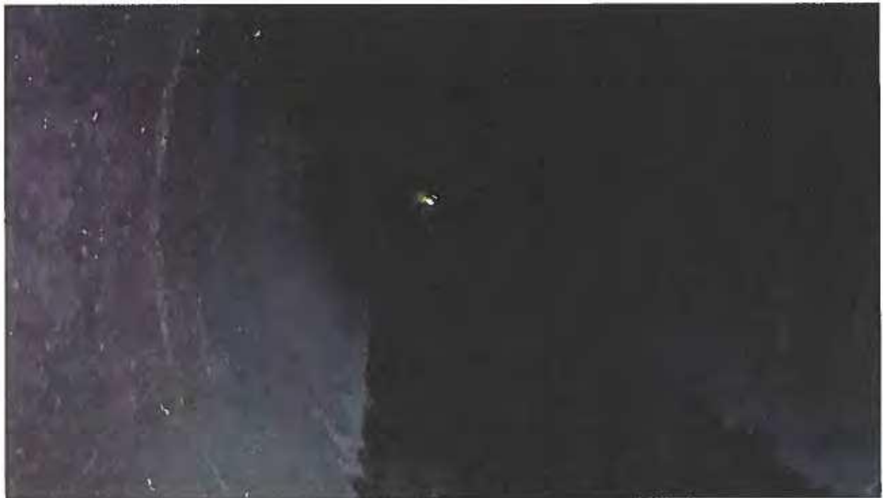
Picture 2. October 18, 2021. The neon green light in the center of the picture corresponds to the water gush coming from the Feeder Canal thru a couple of holes in discharge pipe No.9. The picture was obtained standing next to the corrugated metal panel. Also visible is the stream of backflow in the pipe's barrel.
