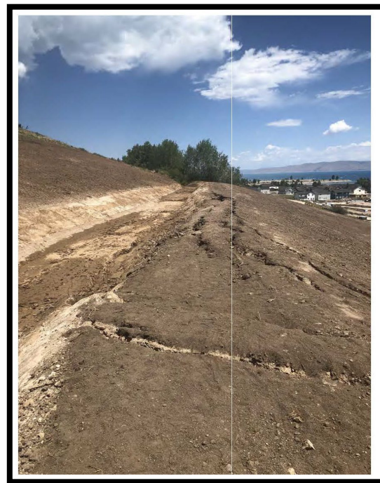
Photo 1 Earthen Canal that is Breaching due to Hillside Encroachment
