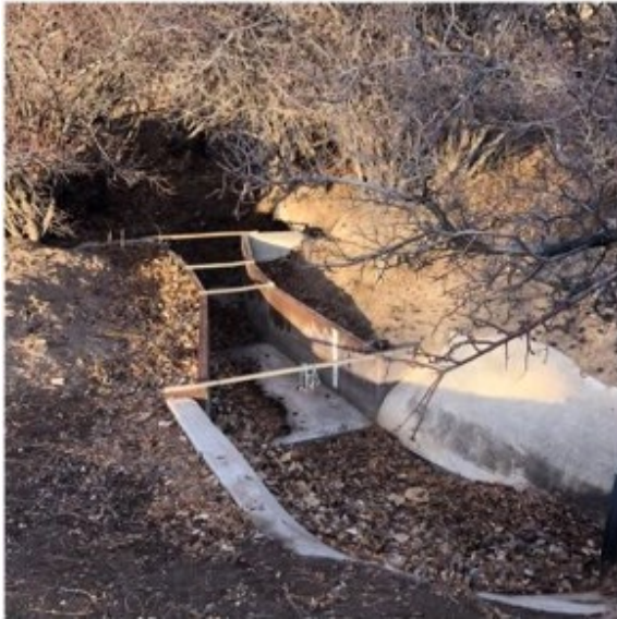
Figure 2: Parshall Flume at Diversion Along Annabella Canal
