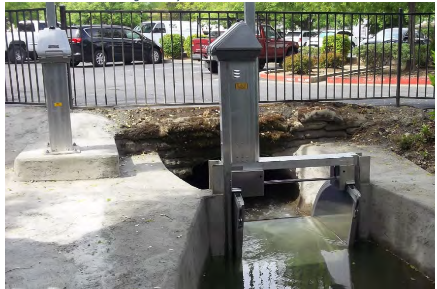
Figure 11. After FlumeGate Installation
