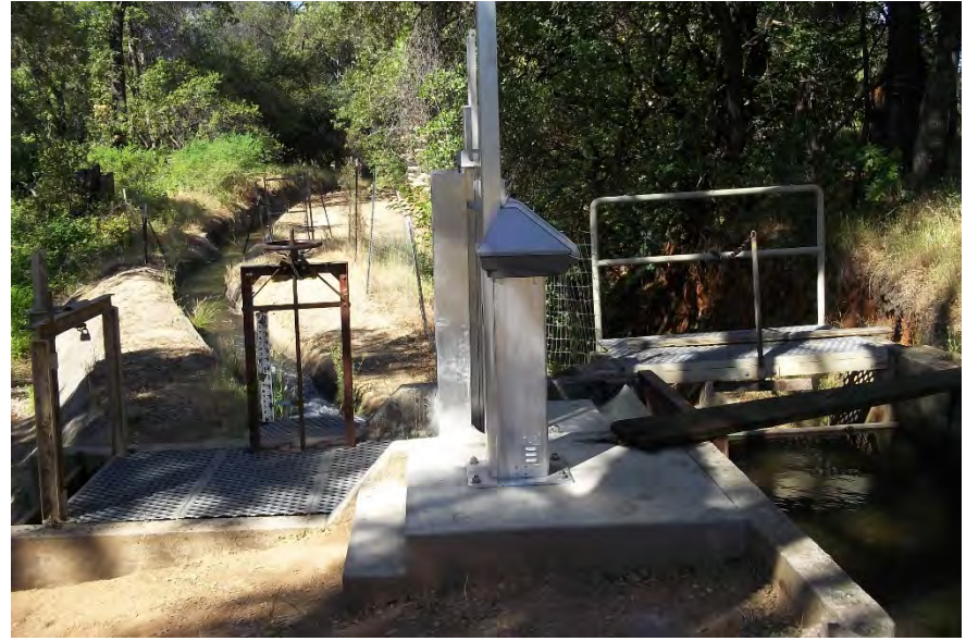
Figure 9. After FlumeGate Installation
