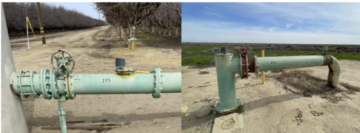
Figure 5. Existing Flowmeters on District Turnouts
