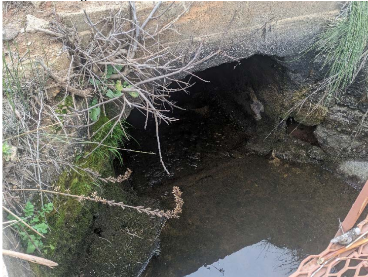
Figure 15. Erosion at West Ditch Headwall
