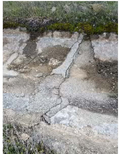
Figure 1. Cracks in Existing Concrete Liner at Teichert Ditch
