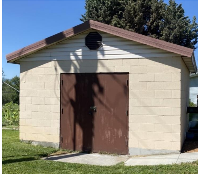
Figure 5: Pump Station to be Removed from Service
