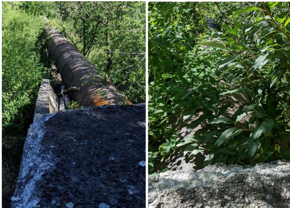
Figure 4: Condition of Black Pipe Supports
