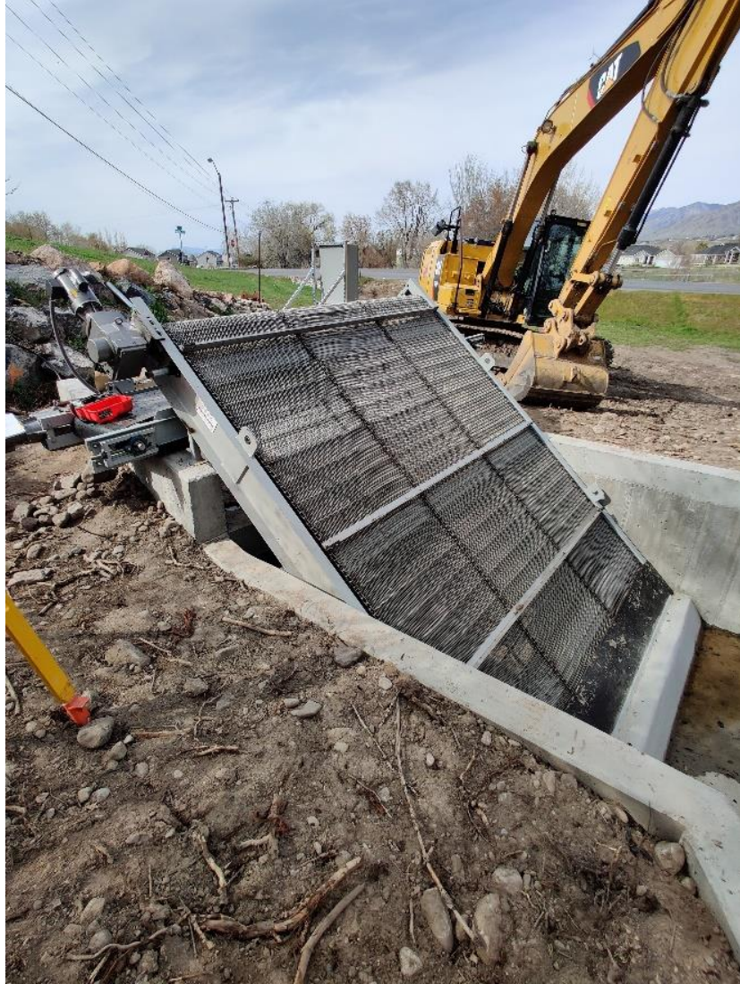
Figure 6: Traveling Wire Mesh Screening Device
