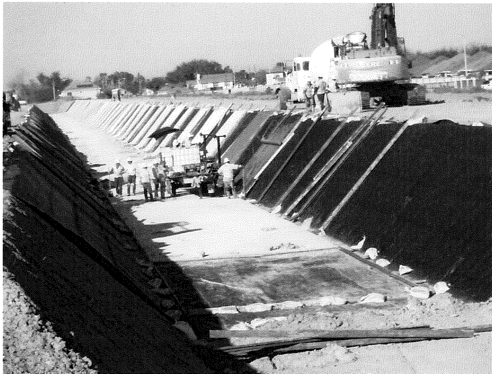
3.3 - Taylor Rd. Canal – This section of canal lining was completed in April of 2022 – The District bid out and contracted for the lining of a .48 mile section of canal with fiber reinforced concrete and Huesker’s Canal 3 liner. The project was completed on time and within budget.
