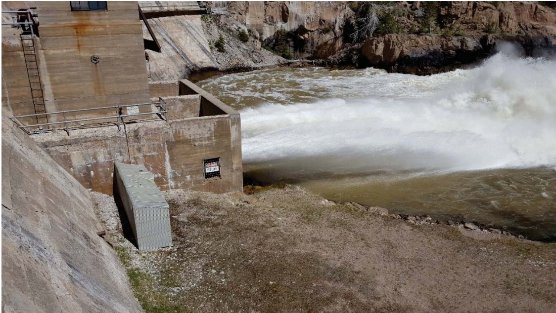
Photo showing typical release from outlet gates; approximately 2,200 cfs.
