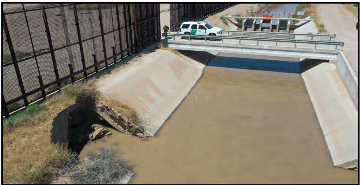
Figure 14. Washout At the U.S.-Mexico Border Fence and Riverside Canal (2020)
