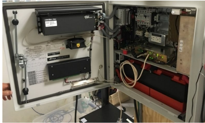
Figure 5. Typical inside of collector cabinet
