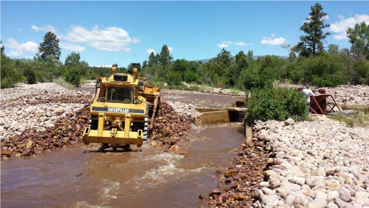
Figure 1: Flooding in 2016 at Existing Structure
