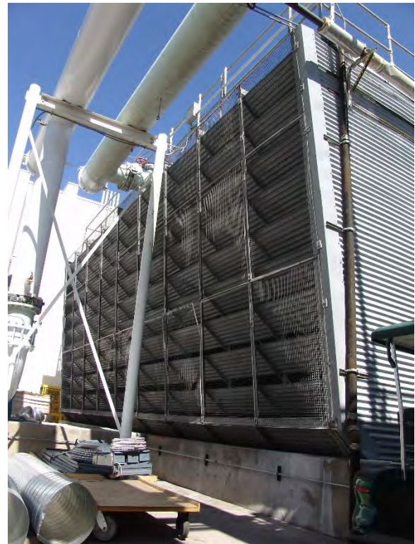
Image: Commercial cooling tower
