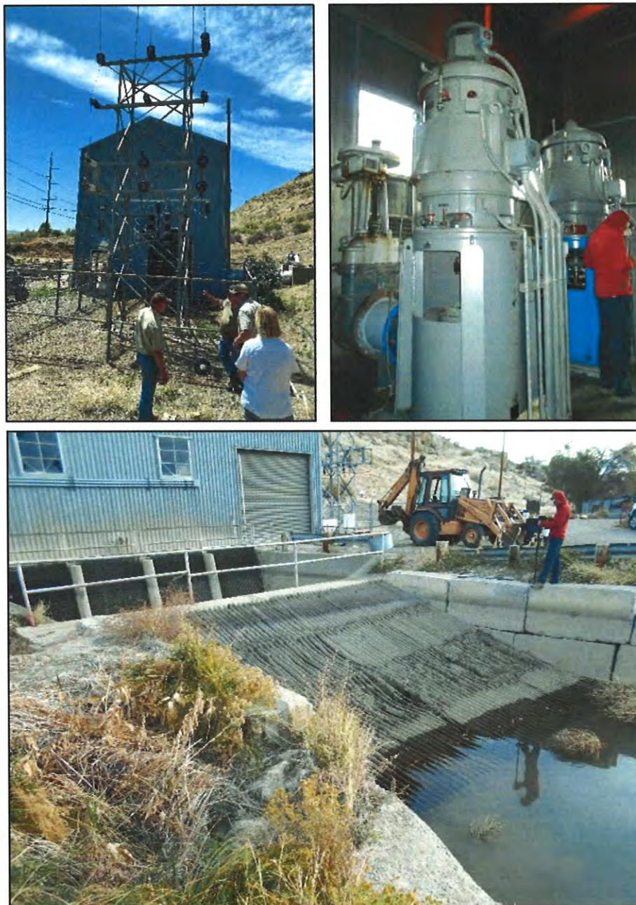
Figure 1.4 OCID Lucerne Main Pump Station
