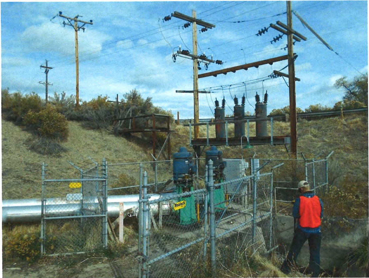
Re-lift Pump Station
