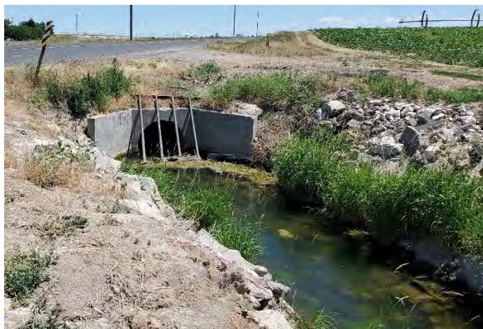
Figure 3 – Typical Irrigation Lateral at Road Crossing
