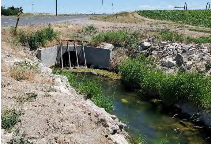
Figure 3 – Typical Irrigation Lateral at Road Crossing
