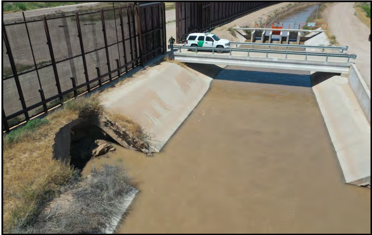
Figure 15. Washout At the U.S.-Mexico Border Fence and Riverside Canal (2020)
