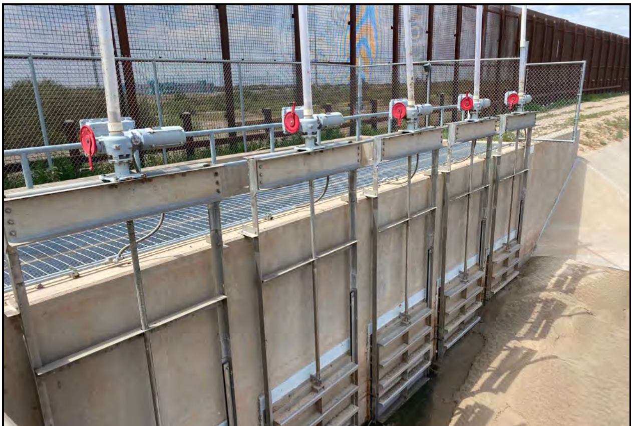
Figure 5. Automated Gates at Riverside Canal Wasteway II
