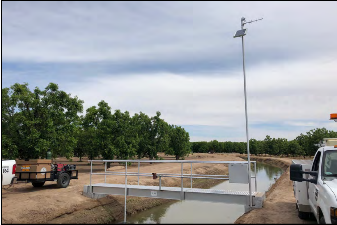
Figure 2. Installed Telemetry Station at an EPCWID1 Lateral (2020)
