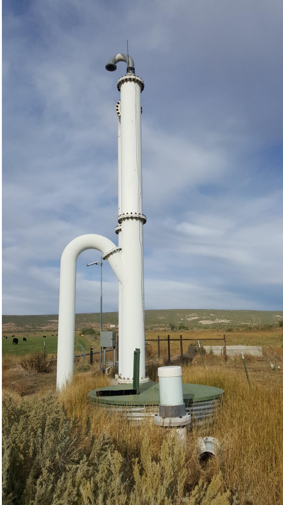
Figure 5: Stand Pipe and Vent at Goliath, Setting Hydraulic Grade for Parry Page Line
