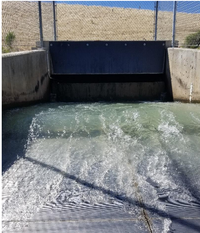
Figure 7: K2 Pipeline Inlet Screen & Baffle of Outlet
