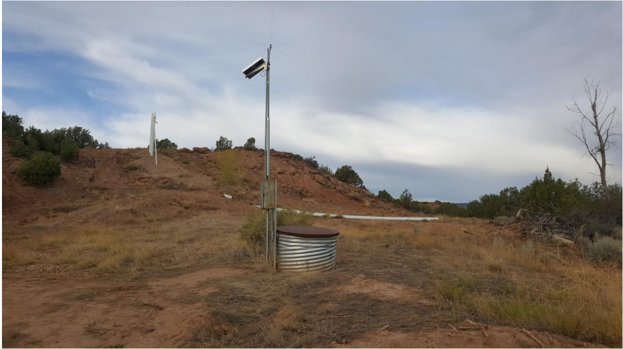
Figure 2: Telemetry on Overflow Pipe at Cottonwood Spill
