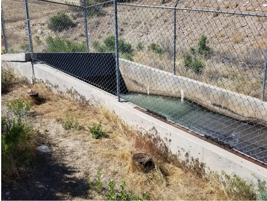
Figure 6: Browns Draw Outlet Structure & Screen
