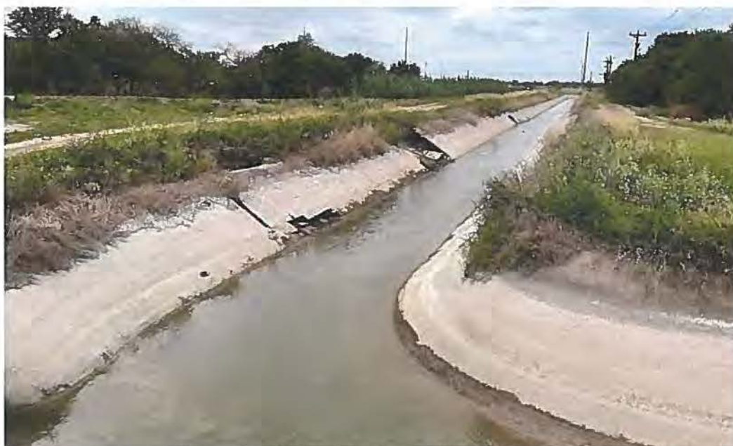
Figure 2.1: Typical Failure of Existing Canal Liner
