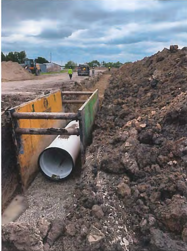
H.I.D.C.C. No.1 – September. 21, 2020; Installation of 48” Closed Profile PVC Pipe -Piping of the Wyrick Canal Phase I, Harlingen, Texas.
