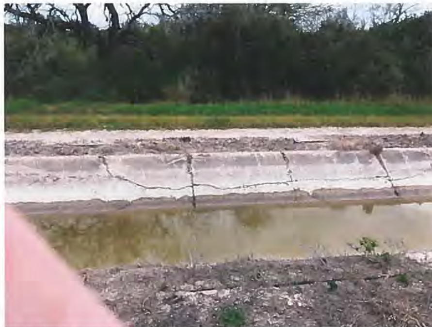
Picture 1. (Background) Visible horizontal crack in the east side slope. Horizontal cracks extend for the entire canal length on both interior side slopes.
