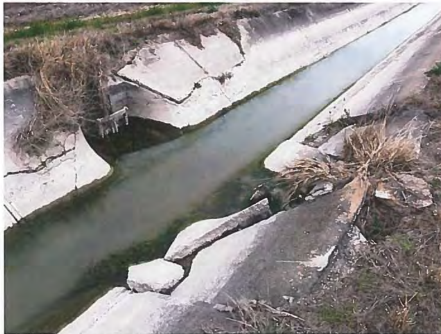
Picture 3 Failure at a service lateral west side slope (right side). The gray to white band in background at approximately 12 inches below the grass line indicates the canal's operational water surface elevation.
