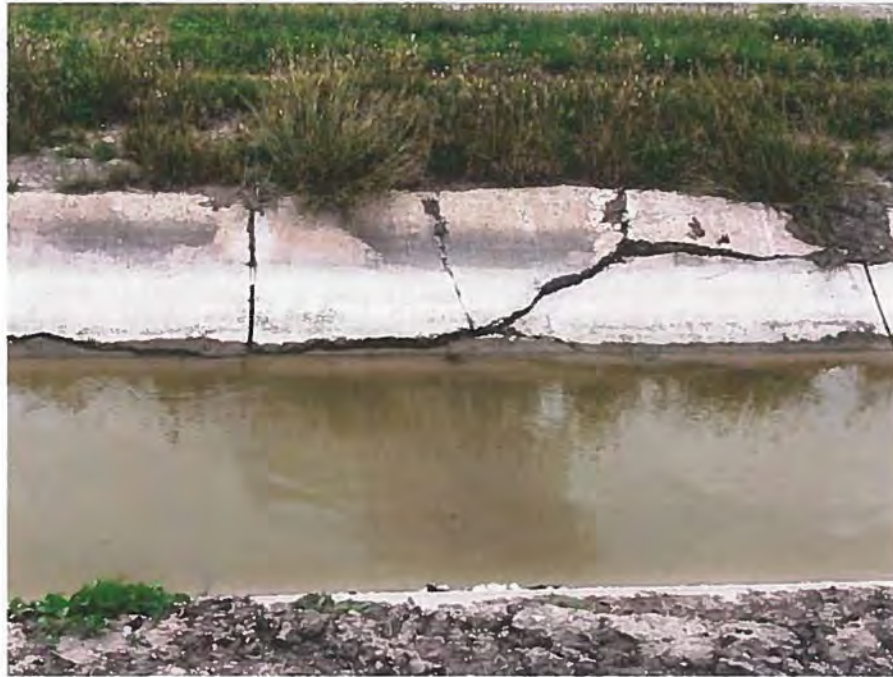
Picture 2 Visible buckling and structural movement.
