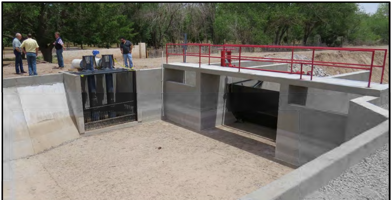
Figure 2: Lift pump on the Eastside Canal conveying water from the head of the Mesilla Dam diversion to the tail end of the Leasburg system
