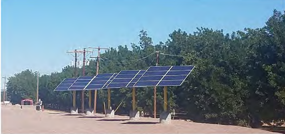
Figure 13: Solar panel array installed by EBID and solar installer at Wasteway 18
