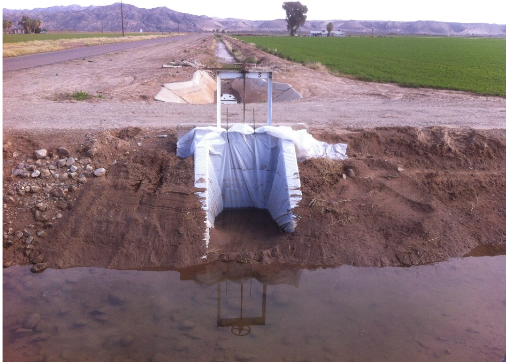
Figure 4. Plastic sheeting sealing off a turnout on 73-19L-1 for seepage test via ponding method.
