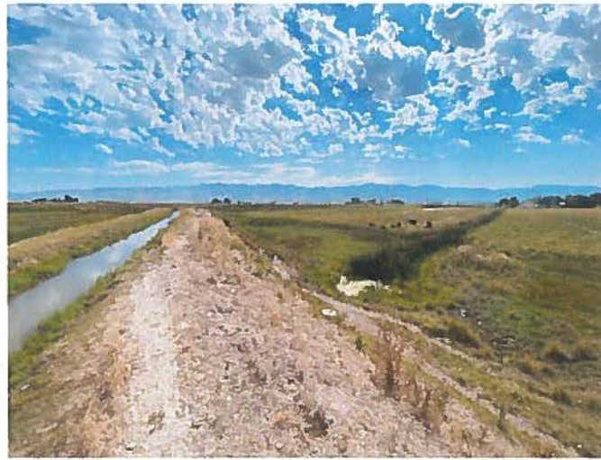
Figure 4: Litz Lateral prior to separation into North and South sections - Illustrating Seepage Loss
