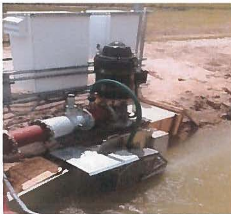
Figure 1: Example of an Existing Personal Irrigation Pumping Station
