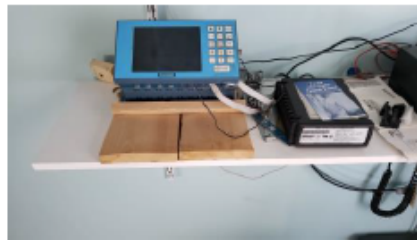
Existing Master RTU Equipment
