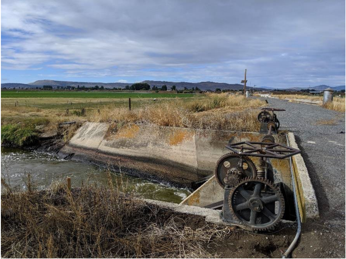
Figure 5 G Canal Head Gates are without automated controls. Flow inaccuracies are common due to human error and inaccurate measurement sensors at the gate.
