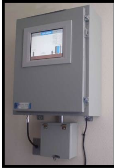
Figure 2 Example of a Modern Master Terminal Unit recommended by Sierra Controls
