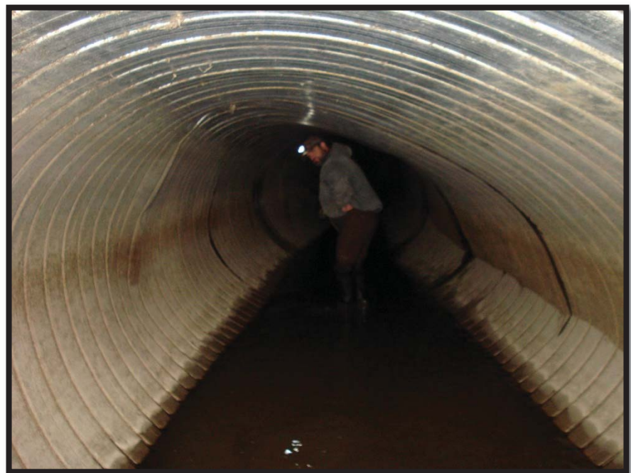
Photo 1 Steel CMP damaged and bent
