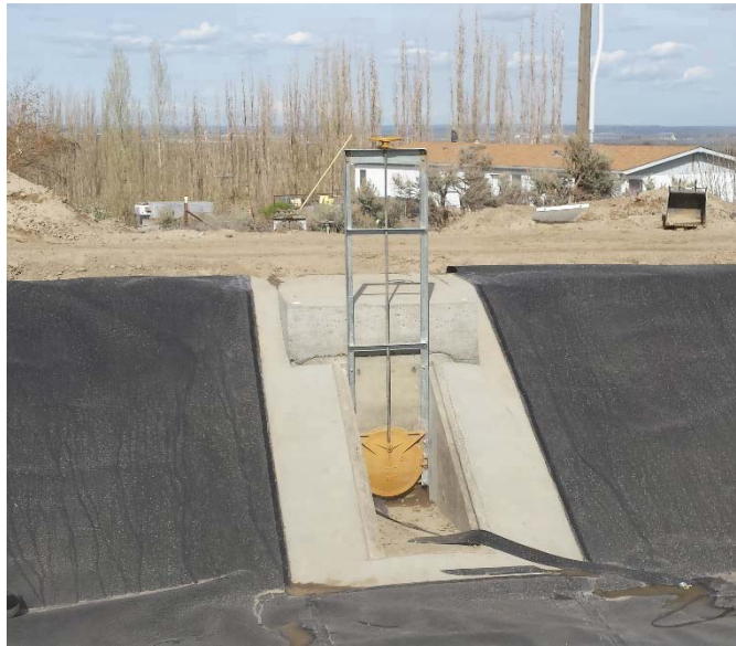
Figure 7. A newly installed turnout slide gate.
