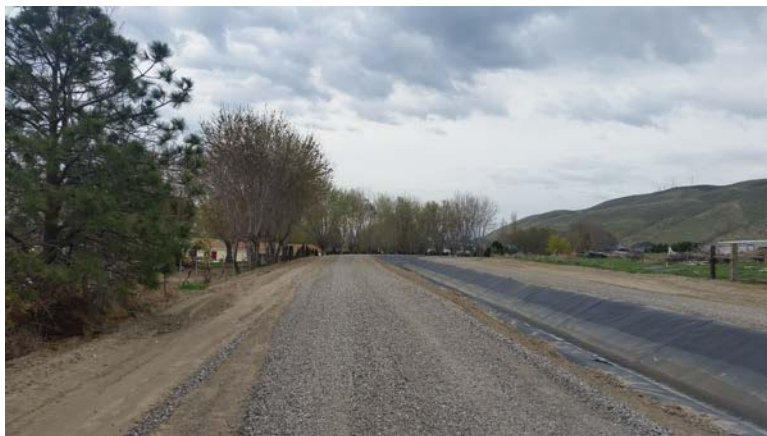
Figure 5. Gravel is picked up and spread by KID crews for new canal roads.
