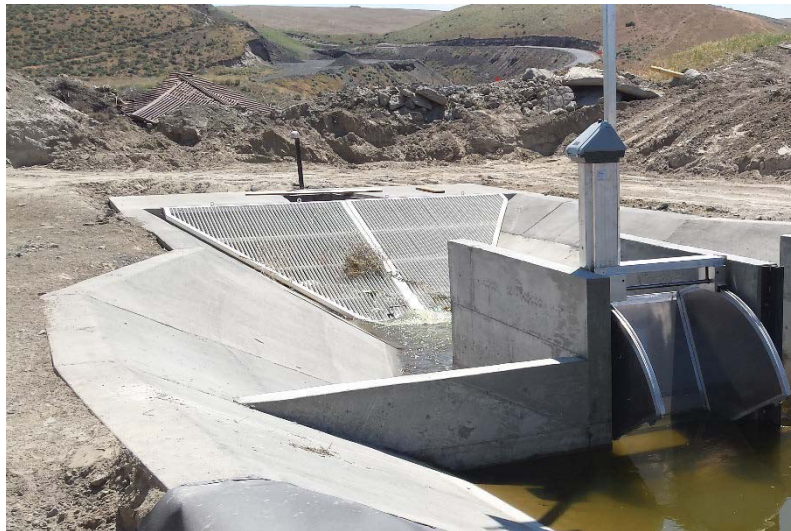
Figure 3. Trash Rack for canal siphon, installed.
