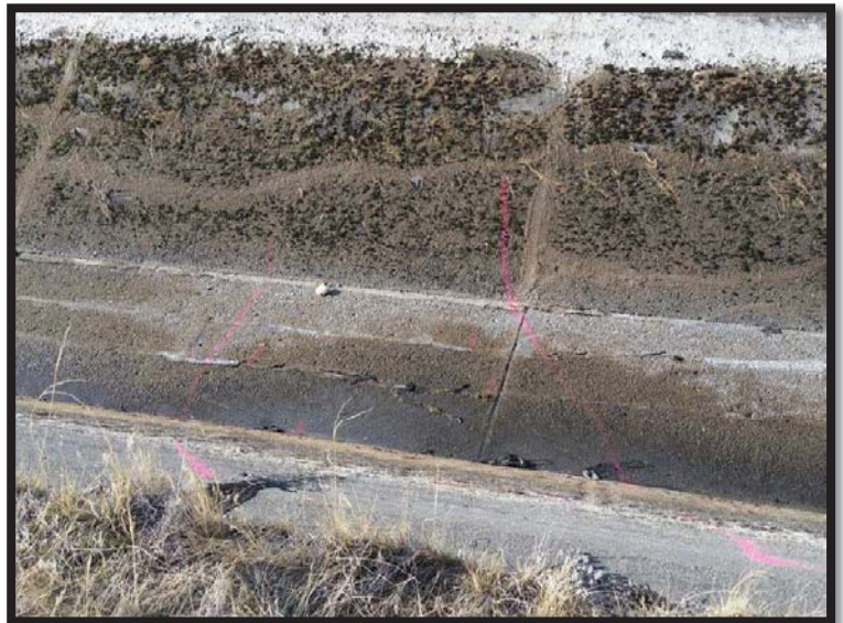
Photo 7 Cracked and broken liner
