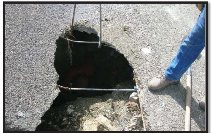
Photo 1 Void within the floor of the Rattlesnake Liner
