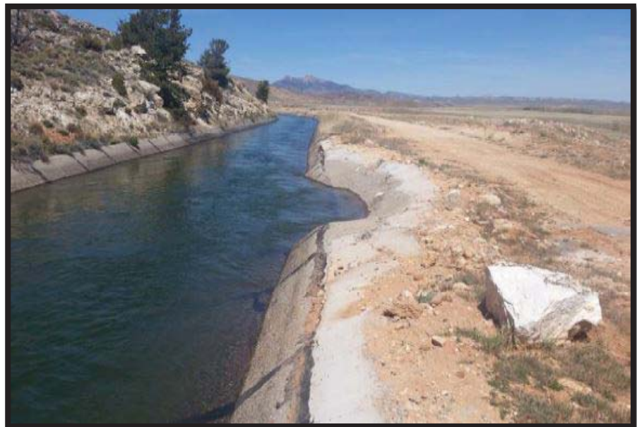
Photo 6 Canal Liner Collapse had to just fill it and go.
