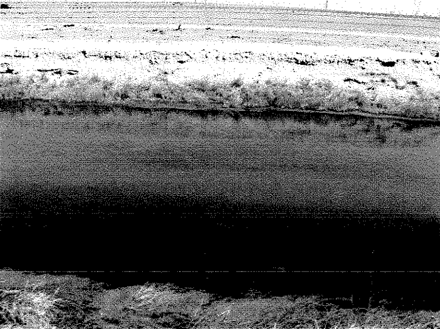
Photograph 2 – Canal Bank Erosion and Aquatic Weed Growth in Existing Earth Canal
