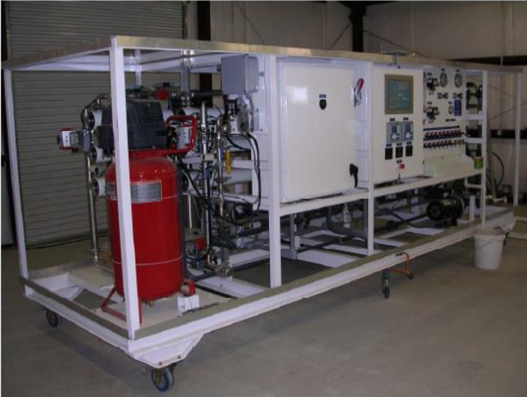
Figure 2: Reverse Osmosis System Photographs
