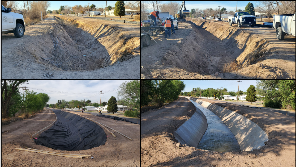
Figure 2. Four Stages of Concrete Lining Work in Phase I of Montoya CL Project
