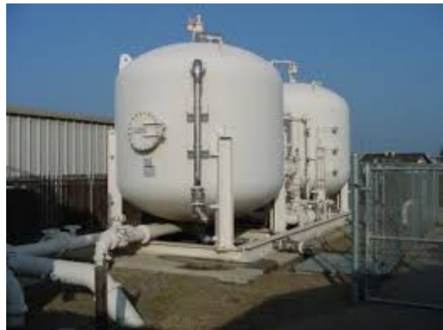
Sanger's water treatment equipment
