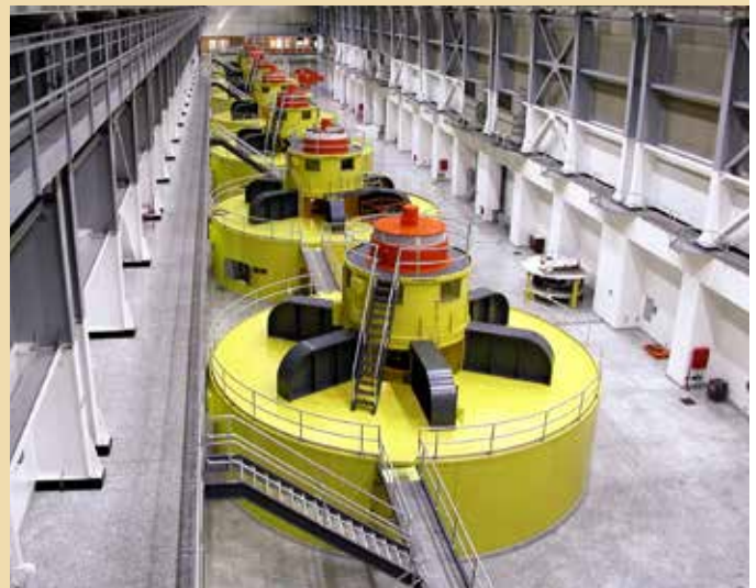
Generators at Glen Canyon Dam, near Page, Arizona.
