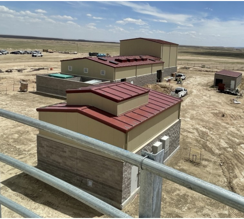
The structures of Tooh Haltsooi Pumping Plant (#4) from the viewpoint atop the newly constructed 1 million gallon water storage tank. Note highway 491 in the background.
