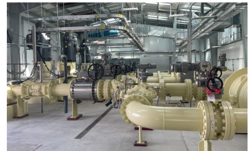
The near completed pipe discharge manifold on the interior of Bahast'ah Pumping Plant.
