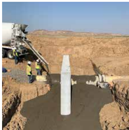
Figure 2 - Backfill of collar 7 days after placement - Block 4c-8. By Hilda Castillo Smith
