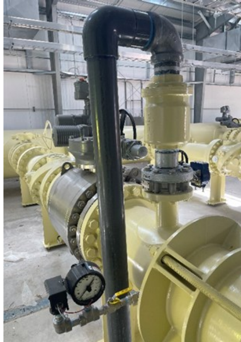
Photo from inside Pumping Plant 4
