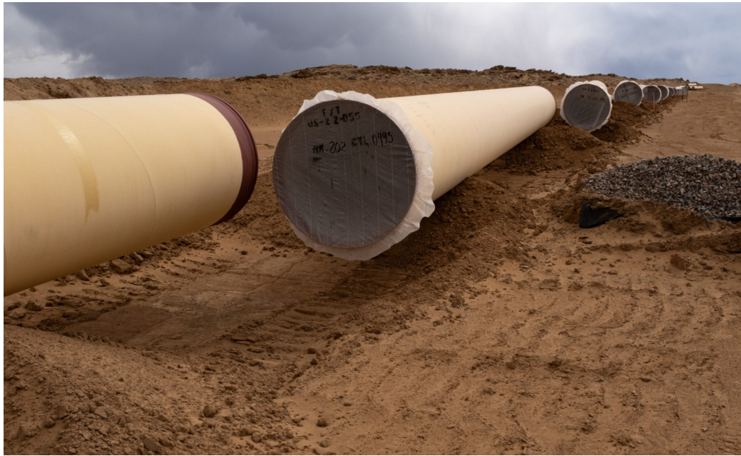
The Navajo-Gallup Water Supply Project, once complete, will deliver water to the communities in the eastern section of the Navajo Nation, southwestern portion of the Jicarilla Apache Nation, and the city of Gallup, N.M., by way of roughly 300 miles of pipeline — transporting water from the San Juan River to those communities. Photo Credit: Jeremy Wade Shockley | The Southern Ute Drum
