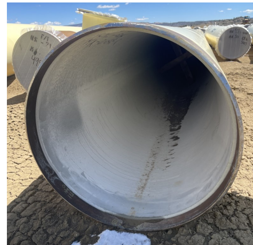
Inside view of 42-inch steel pipe, located at the Sanostee Chapter area Reaches 4A/4B
