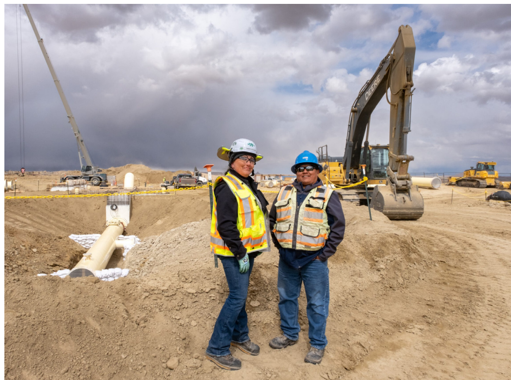
Coordinating on the Navajo-Gallup Water Supply Project, Bureau of Reclamation Materials Engineering Technician, Lalena Weasel and Archer Western Construction Quality Control Manager, Timber Loveland stand together on-site Thursday, March 7, where construction is underway for a new pumping plant facility south of Shiprock, N.M. Photo Credit: Jeremy Wade Shockley | The Southern Ute Drum
