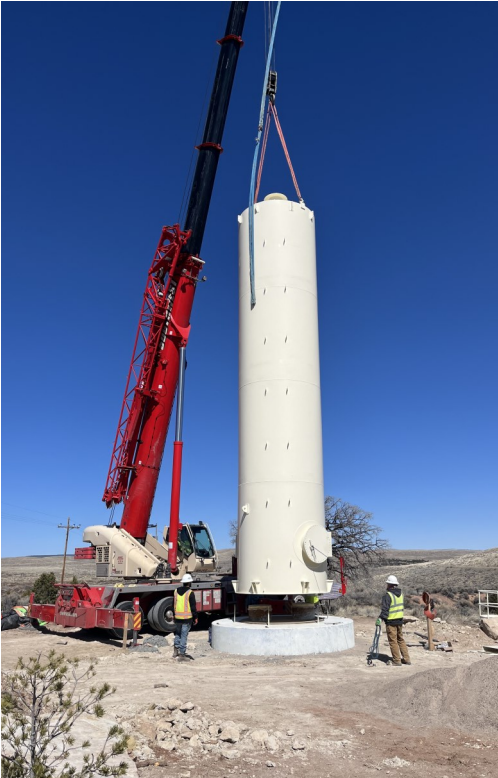
Crews use a crane to lower the McKinley Surge Tank onto the foundation on Code Talkers
