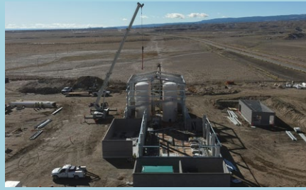
Tank installation at Pumping Plant 4
