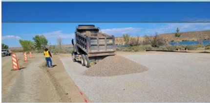
Site Preparation for the Pilot Study Water Filtration System of the San Juan River
