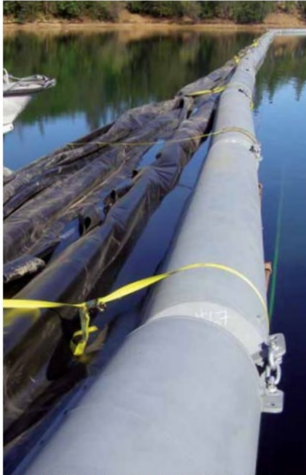
FIGURE 8 Metal floats in place and curtain ready to be anchored to the river bottom by 800-lb weights Photo: Bureau of Reclamation
