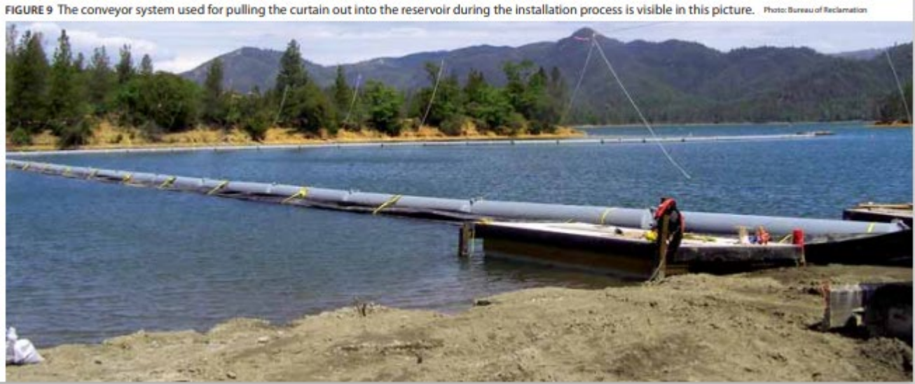
FIGURE 9 The conveyor system used for pulling the curtain out into the reservoir during the installation process is visible in this picture. Photo: Bureau of Reclamation
