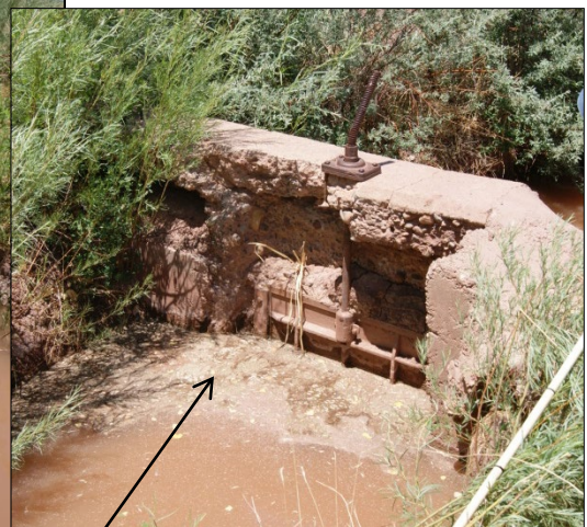
East Ditch gate current condition. Located 100 ft . (est.) from bend in canal in photo at left.
