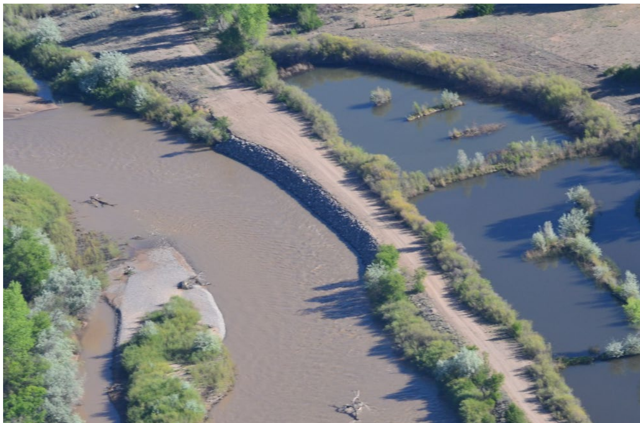
Figure 6: Photo looking north toward completed bank stabilization work at Ohkay Owingeh Pueblo (Reclamation, 2024)
