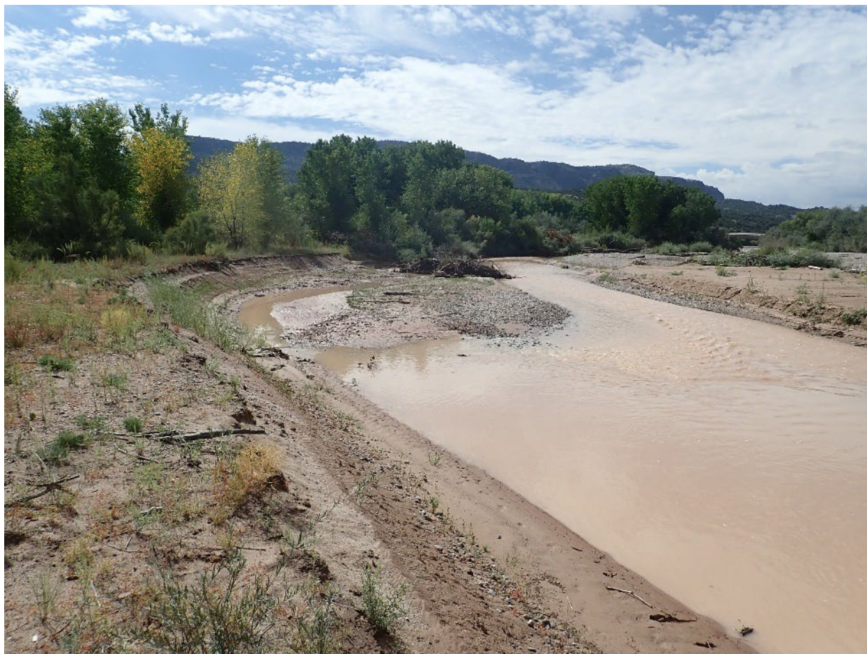
Figure 8: Photo taken September 17, 2024, looking downstream toward the eroded area.
