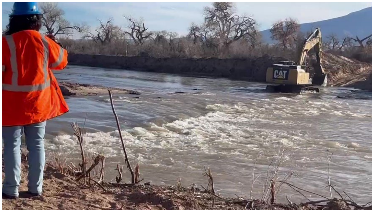
Figure 11. Excavator crossing the Rio Grande at a constructed riprap crossing at RM 199.
