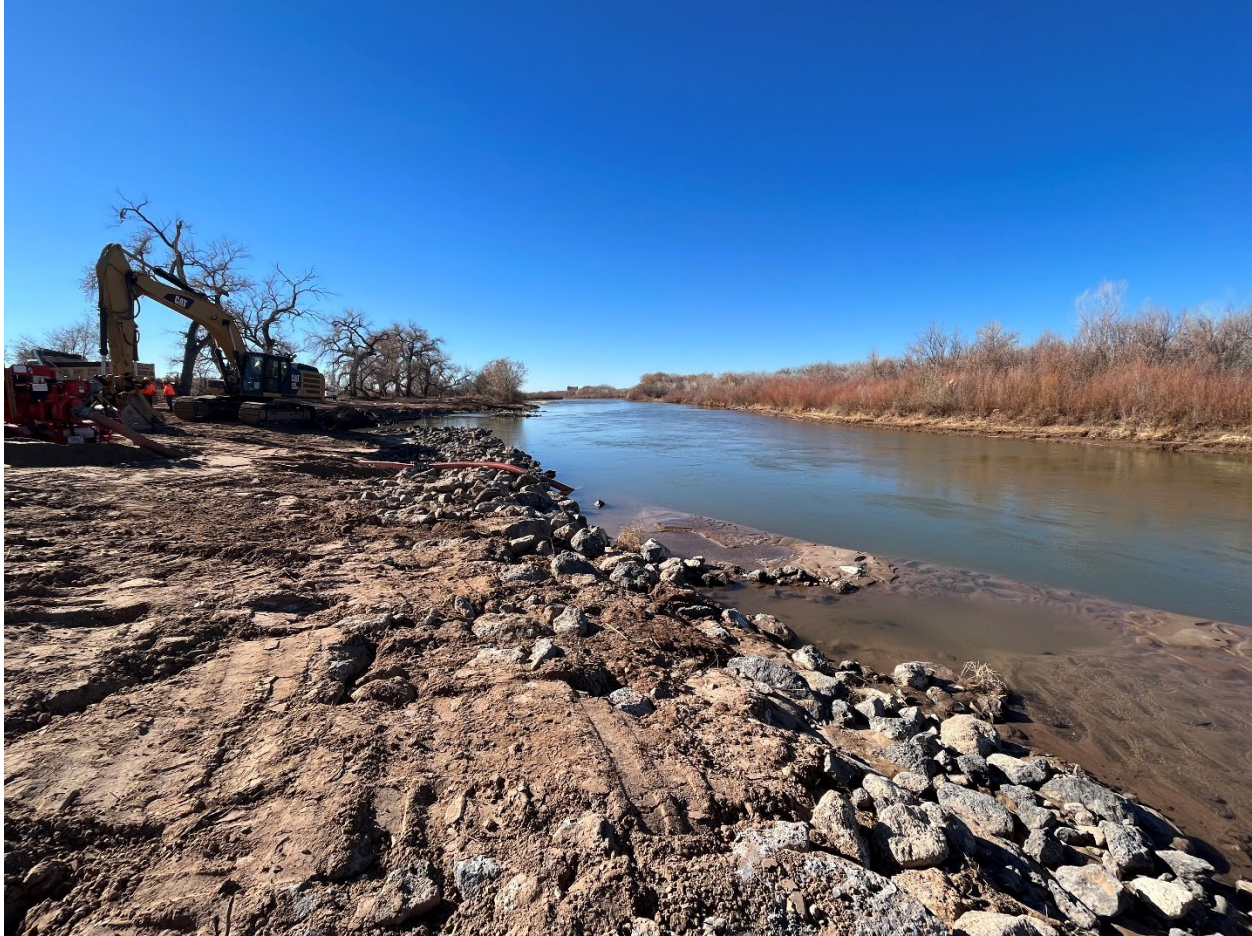
Figure 6: Looking downstream at placement of riprap for longitudinal stone toe protection on the eastern bankline; scour hole is visible in the distance (Reclamation)
