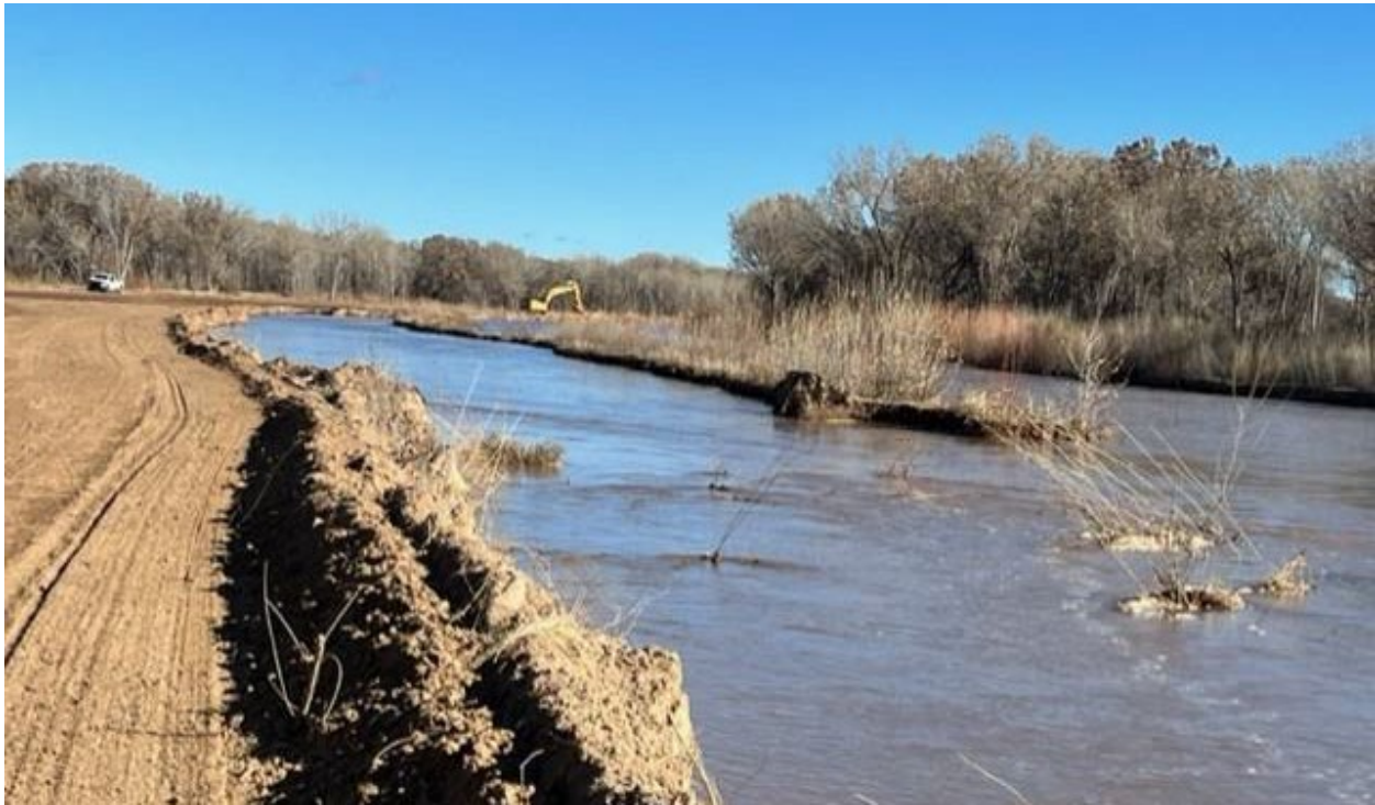
Figure 14: Channel maintenance work at the knickpoint site on the BDA Lower Realignment Project (Reclamation)
