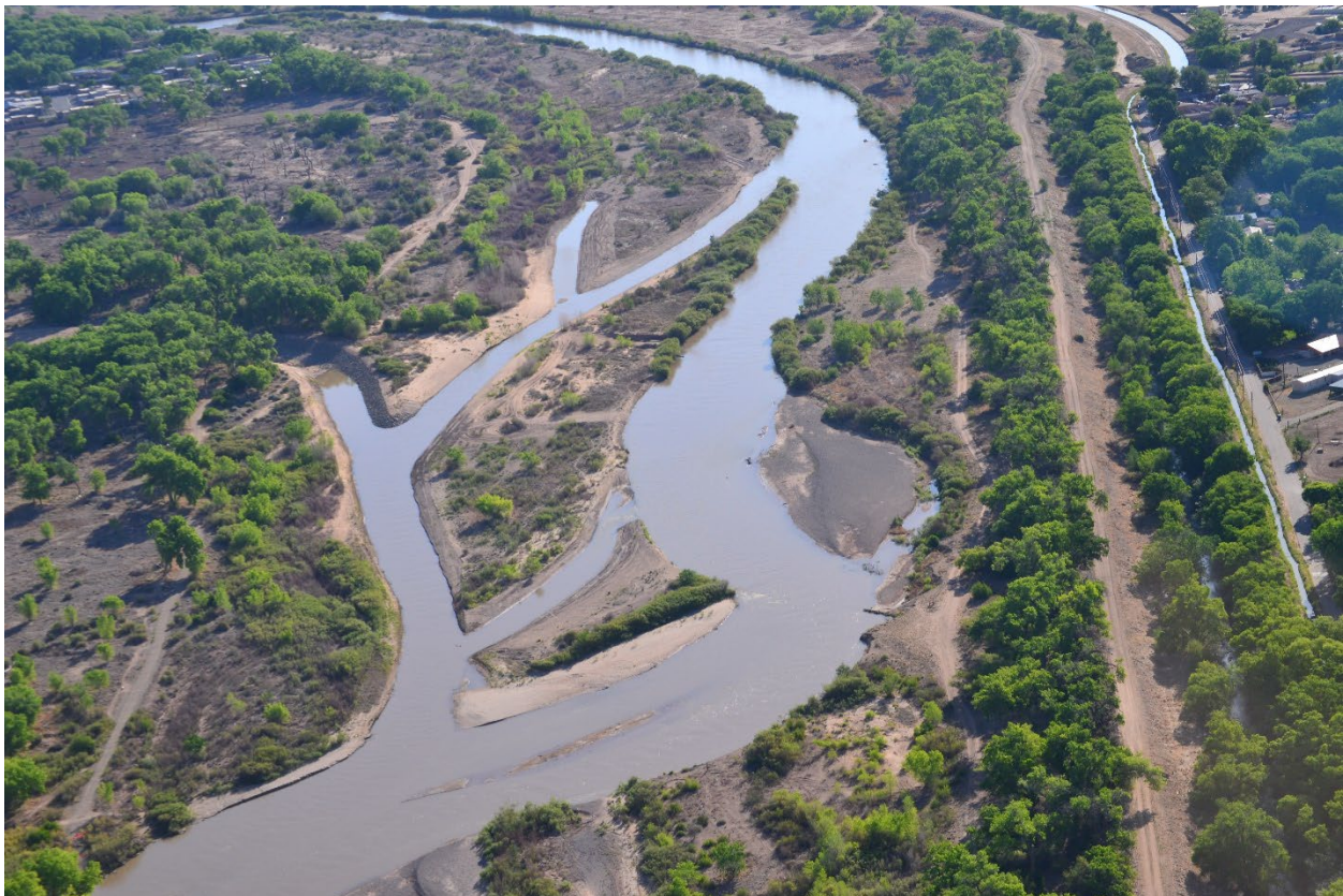
Figure 7: Construction of new side channels on the western floodplain of the Sandia Priority Site (Reclamation)
