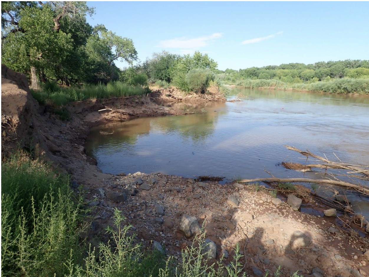
Figure 5: Looking downstream at Santa Ana RM 205.8 east bankline bendway weirs and repairs (Reclamation)
