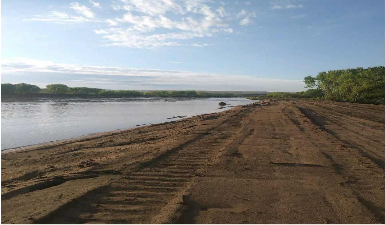
Figure 13: View of realigned Rio Grande channel on the BDA from the west bank following summer monsoonal flows (Reclamation)
