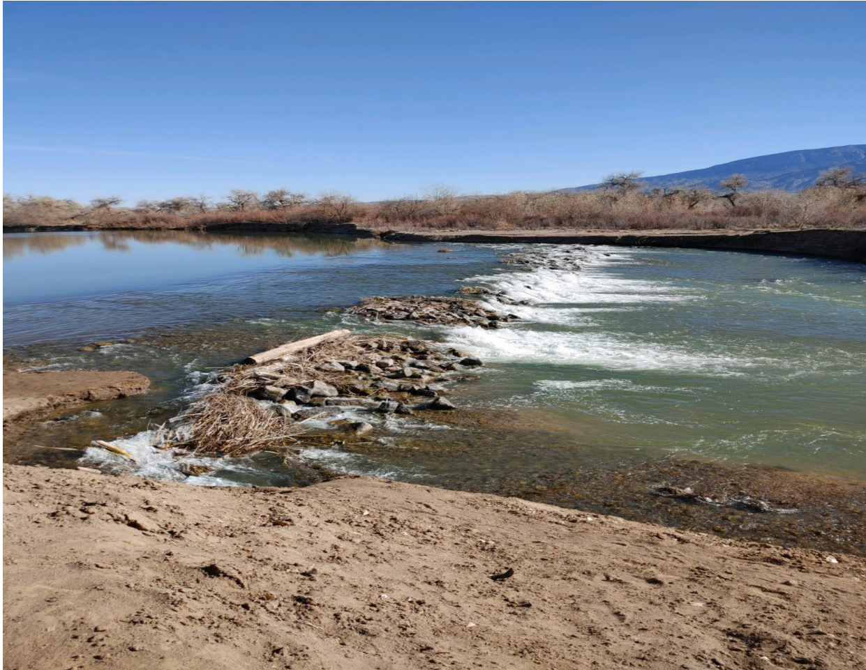
Figure 9: Looking east at the Corrales Siphon and the 2020 riprap protection placed downstream of the siphon (Reclamation)
