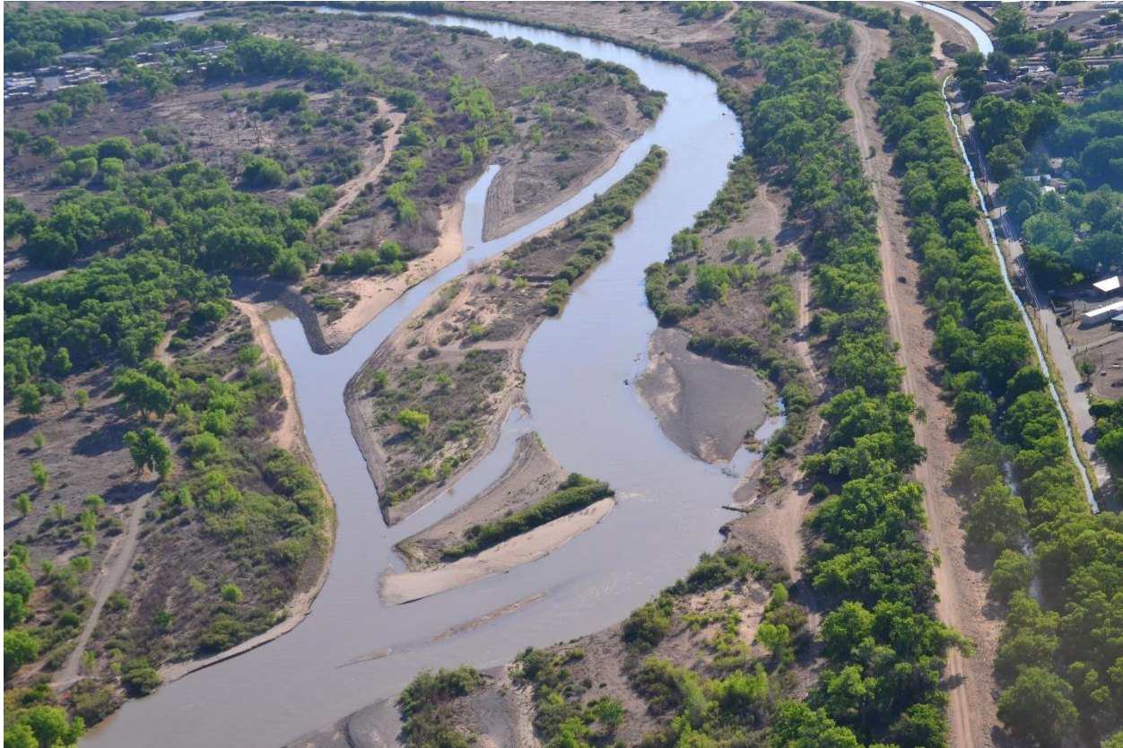
Photo 2: Construction of new side channels on the western floodplain of the Sandia Priority Site (Reclamation, 2021)
