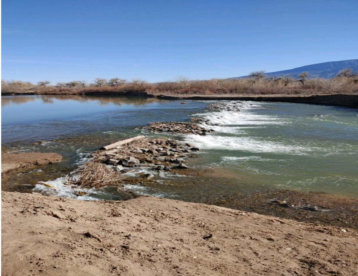
Photo 3: Looking east at the Corrales Siphon and the 2020 riprap protection placed downstream of the siphon (Reclamation, 2021)
