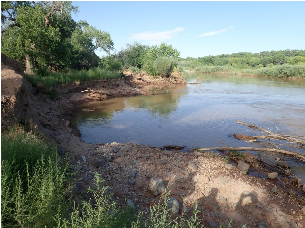
Photo 1: Looking downstream at Santa Ana River Mile 205.8 east bankline bendway weirs and bankline repairs (Reclamation, 2021)
