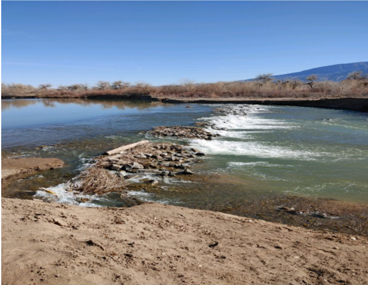
Photo 3: Looking east at the Corrales Siphon and the 2020 riprap protection placed downstream of the siphon (Reclamation photo)
