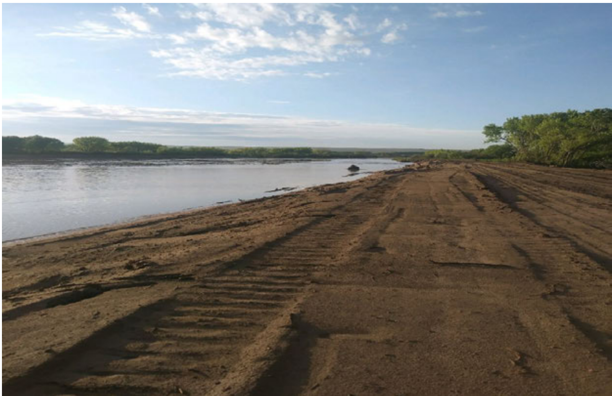
Photo 6: View of realigned Rio Grande channel on the BDANWR from the west bank following summer monsoonal flows (Reclamation photo)
