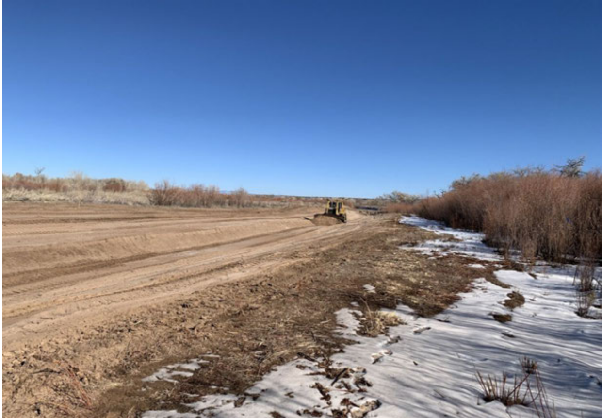
Photo 2: Construction of a new side channel on the western floodplain of the Sandia Priority Site (Reclamation photo)
