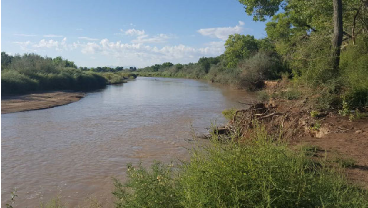
Photo 3: New erosion in the RM 199 project area. Photo is looking downstream immediately below Corrales Siphon. (9/11/2019)
