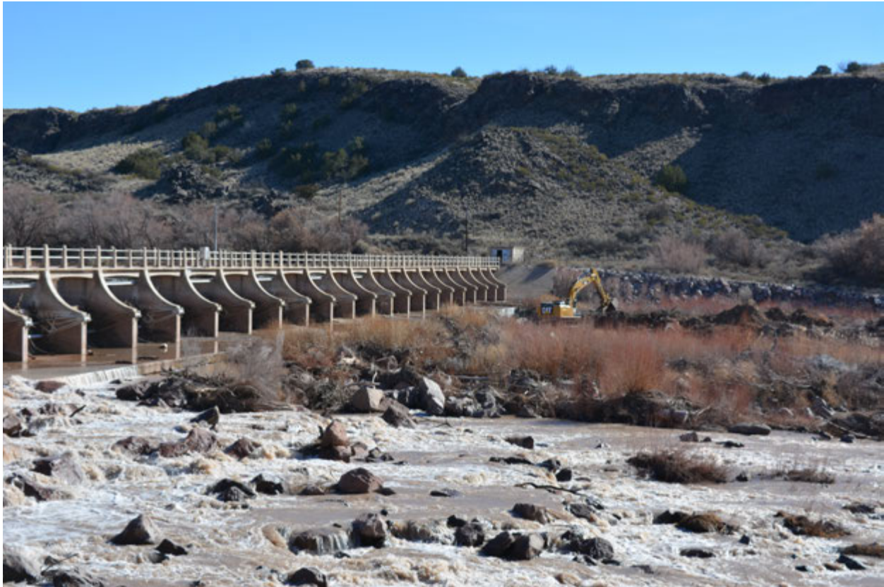
Photo 5: Construction work has begun to rehabilitate the rock ramp below San Acacia Diversion Dam's concrete apron to create a 10% design slope on the ramp as it transitions from the dam's headworks onto the downstream river channel (flow about 500 cfs; January 2019)
