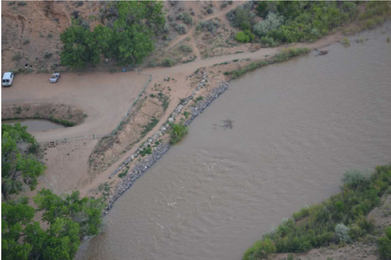
Photo 3: View looking downstream at the Corrales Siphon and the 2016 riprap protection placed downstream of the siphon
