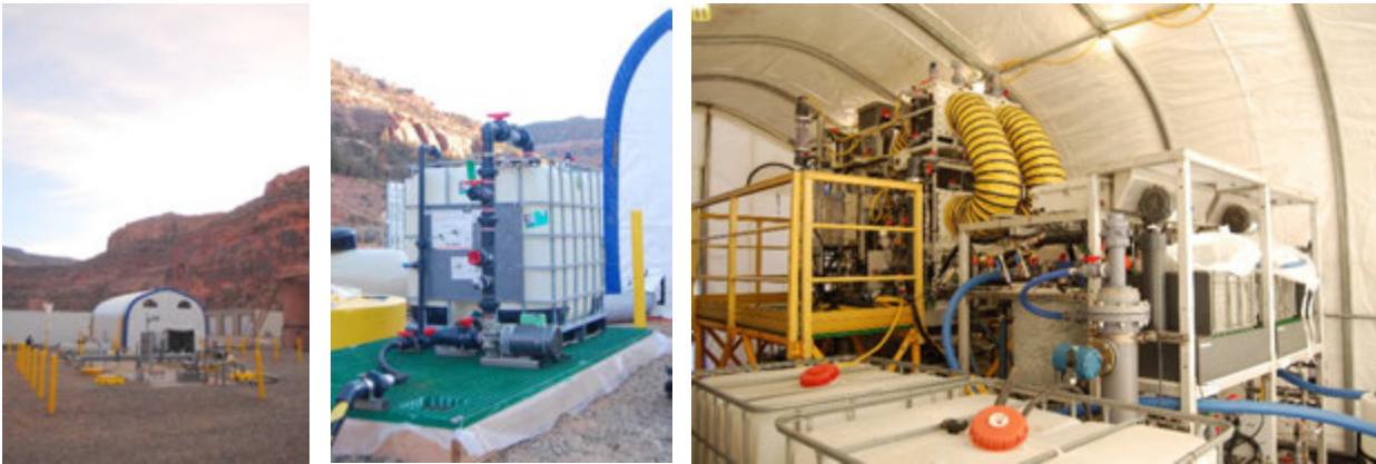
Figure 2: SaltMaker Pilot at Site (left), H 2 S Pretreatment Skid (middle), SaltMaker Pilot (right)
