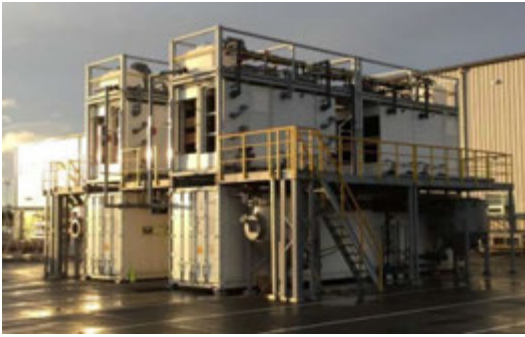
S100 SaltMaker Plant 100 m 3 /day freshwater removed capacity
