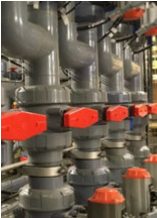
Pipework UPVC and CPVC
