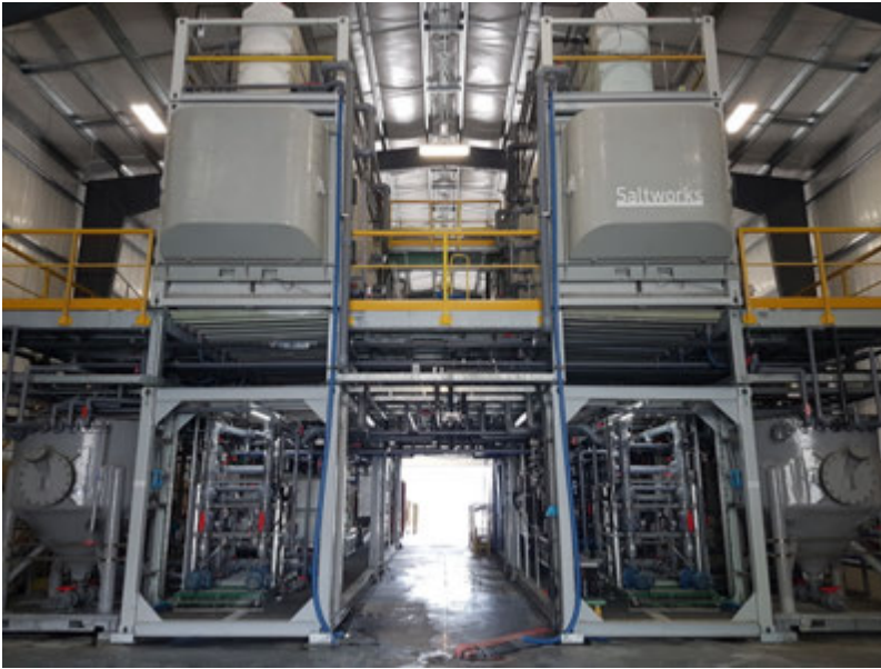
Modular SaltMaker Plant Built into Standard ISO Frames
